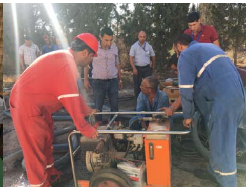
Test of Power Pack
